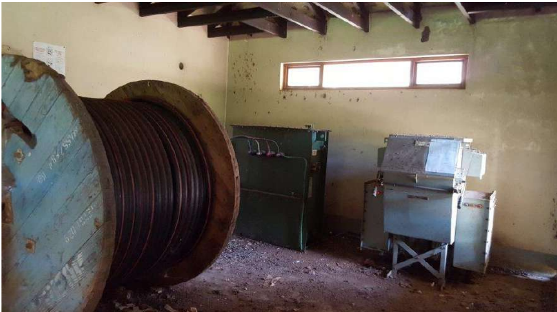
Existing transformer at Bhangazi substation
