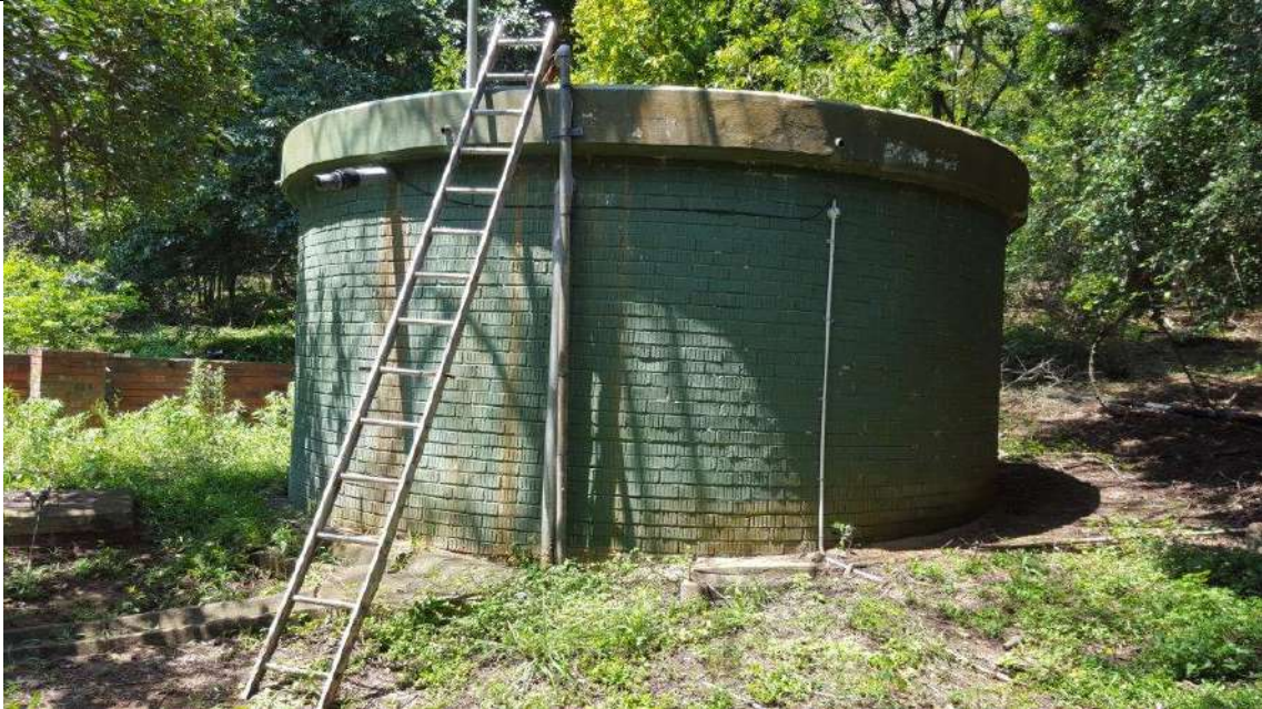
Existing reservoir (70kl) at water pump station fed from the existing borehole
