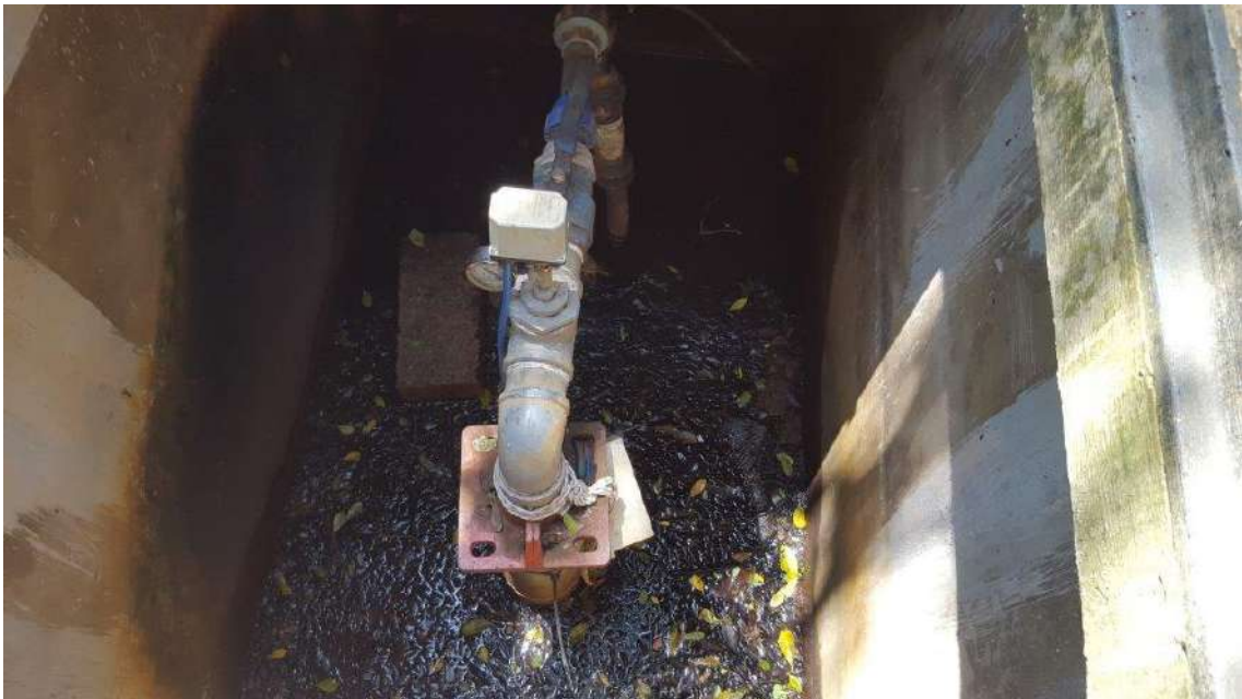
Borehole with submersible pump at Bhangazi site
