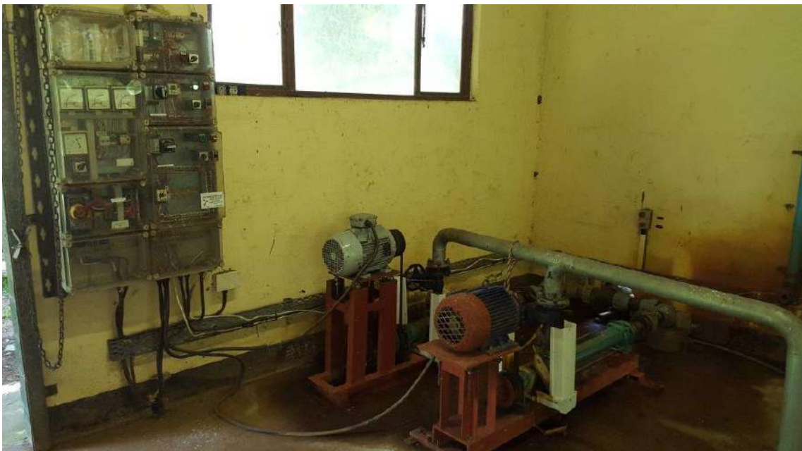
Existing water pumps at Bhangazi transferring raw water to reservoir at Cape Vidal
