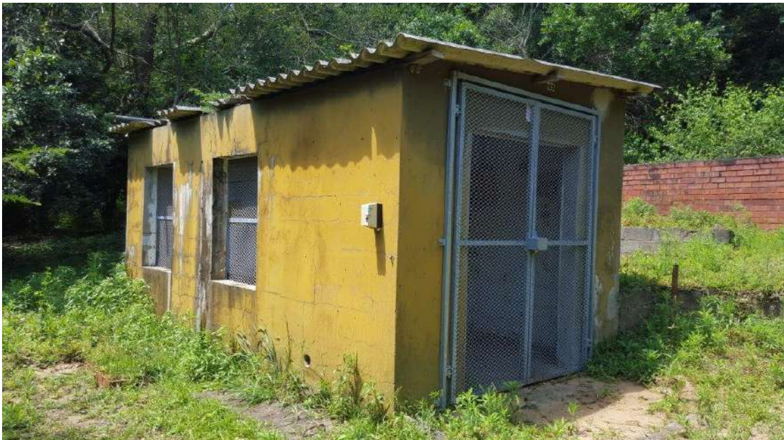
Standby generator at the water pump station serving the MTN tower
