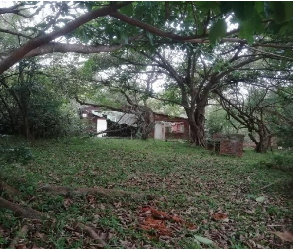
Figure 11 Proposed senior staff camp on old, disturbed areas with building in a state of disrepair, surrounded by figs and white stinkwoods
