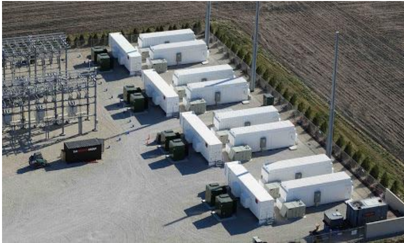
FIGURE 8-7 A STOCK IMAGE OF A SIMILAR DEVELOPMENT WITH AN ON-SITE SUBSTATION AND BESS
