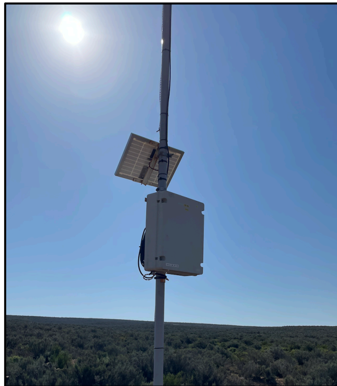
Figure 5: System G on a 10 m mast at the proposed Khoe WEF
